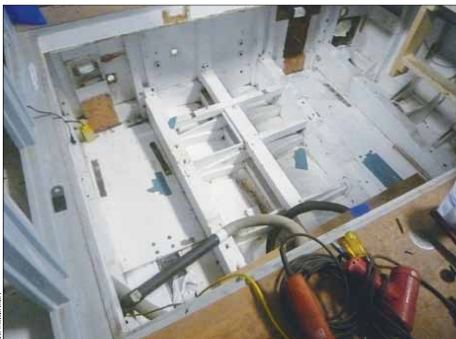
The engineroom early in the rebuild, just after the conventional V-drive Cummins diesels and running gear were removed. Engine beds, hull bottom, and most of the structural members pictured here were replaced in order to accommodate the new engines.
