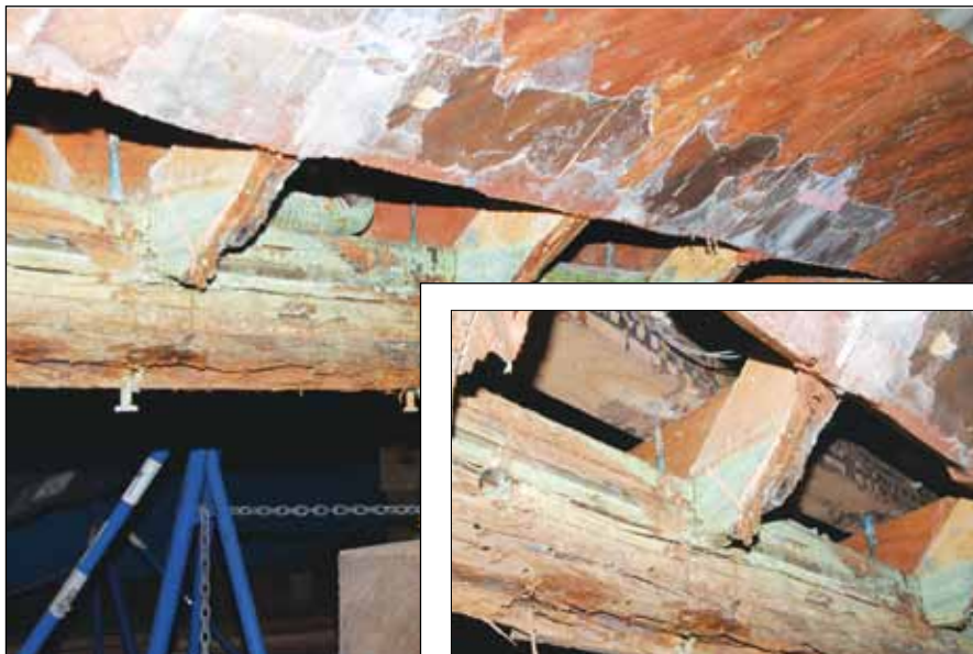
Cutting back the garboard area forward of the engineroom revealed more deterioration in the frames, floors, and full-length laminated keel and stempiece. That clinched the decision to replace the entire double-diagonal planked bottom forward of the engineroom.
